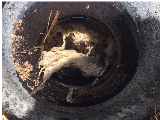
City of Cascade WW Lift Station - Lakeshore Pump alarm triggered a shutdown of the pump due to the presence of a large COTTON MOP HEAD . Picture taken Fall of 2019.
